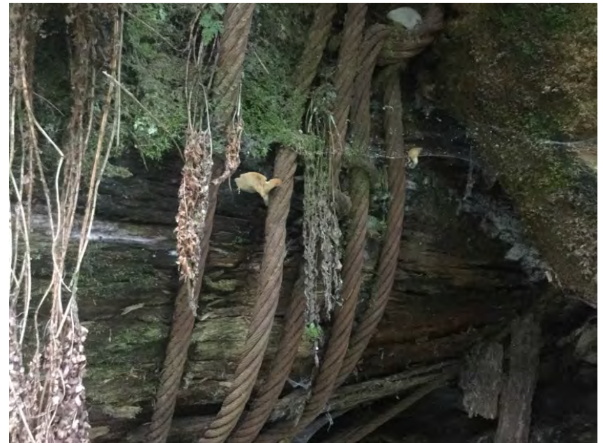
Stringer 1 Small Fungal Growth
