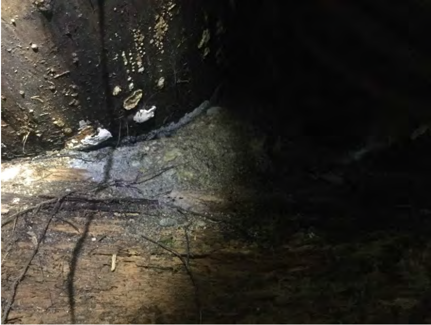
Stringer 2 Fungal Growth
